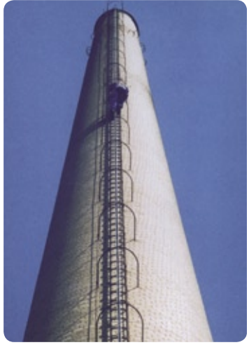
Chimney with retrofitted guide rail
